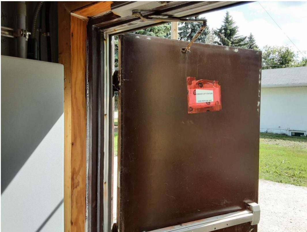
Metal, Brown over grey, V0002(Lead-containing), Exterior of Building (Location #: 6)
