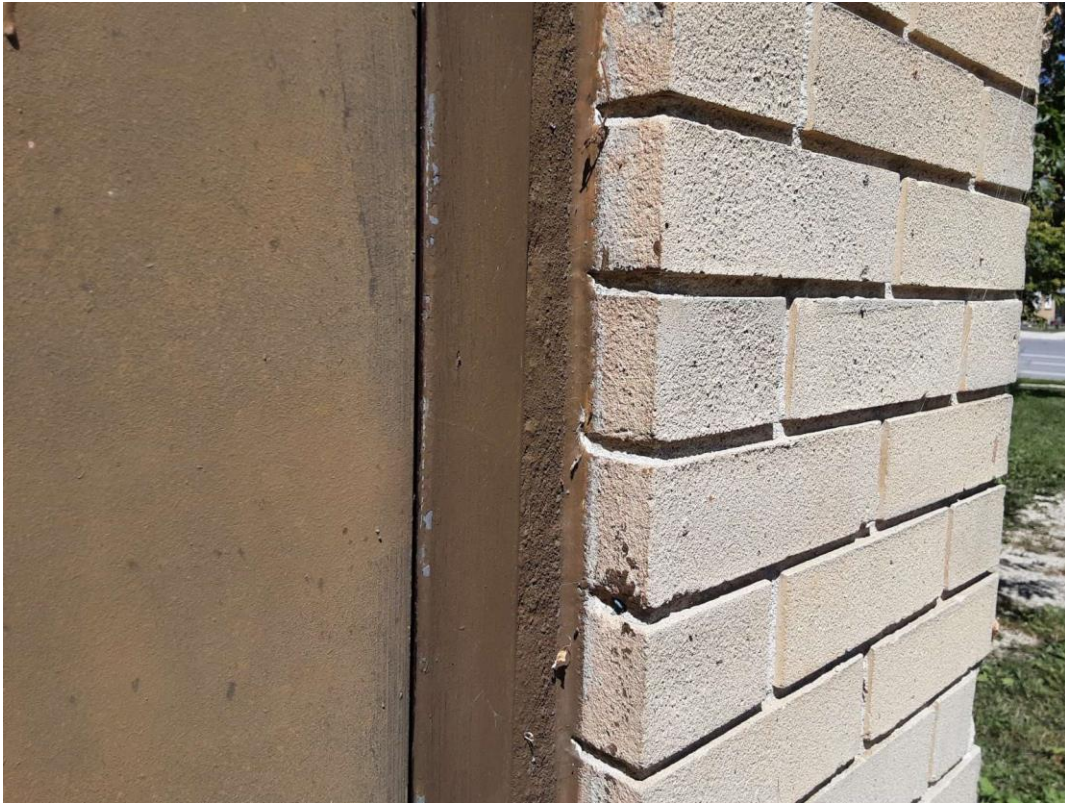
S0003A (None), Other, Caulking, Exterior of Building (Location #: 6)
