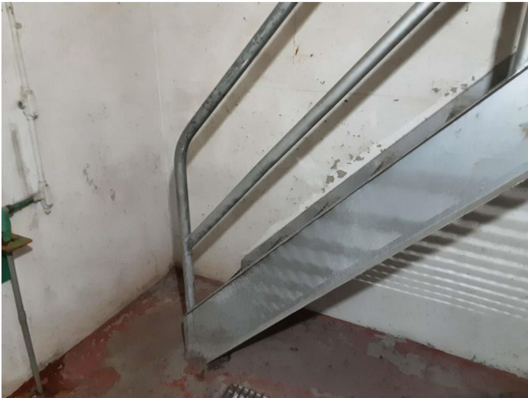
Motor Room (Location #: 4)
